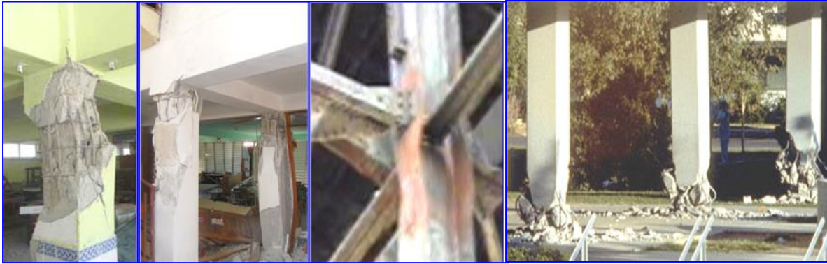
Figure 4. Weak column-strong beam failure [5]
